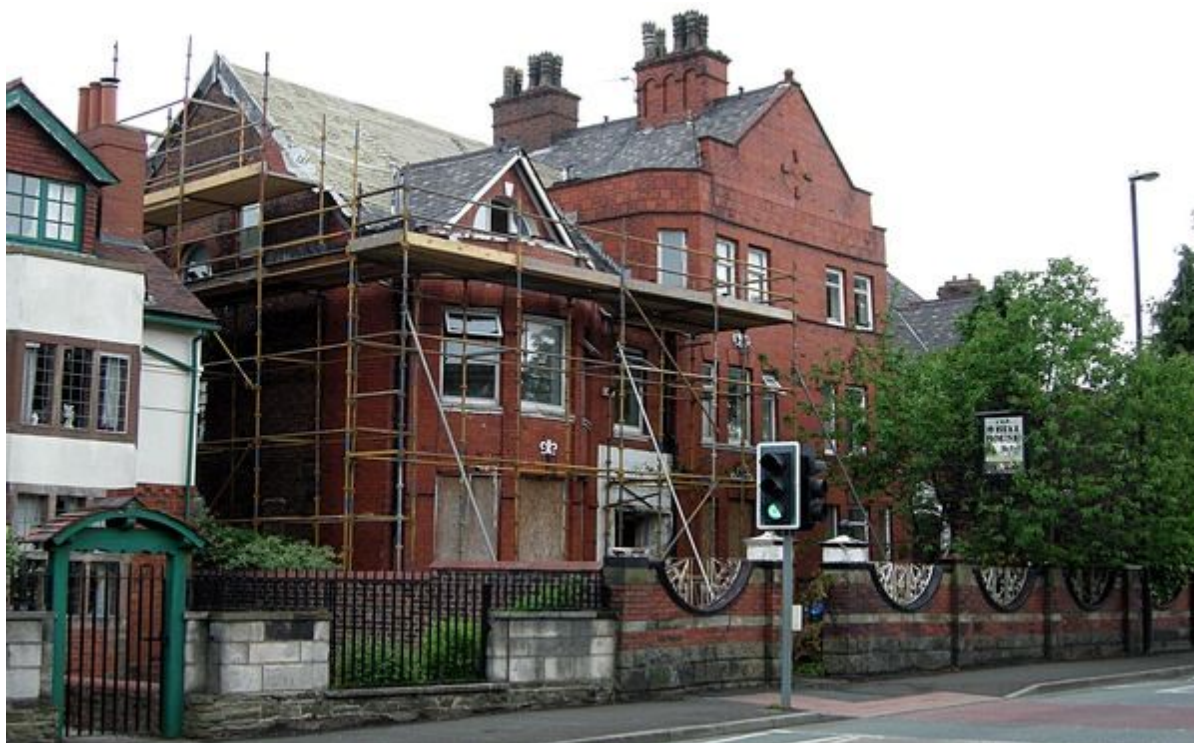
Plate 23 With the input of Rochdale M.B.C. conservation officer, Hillcrest was reroofed and masonry repairs undertaken to the bow window in 2008. Photo: David Morris
